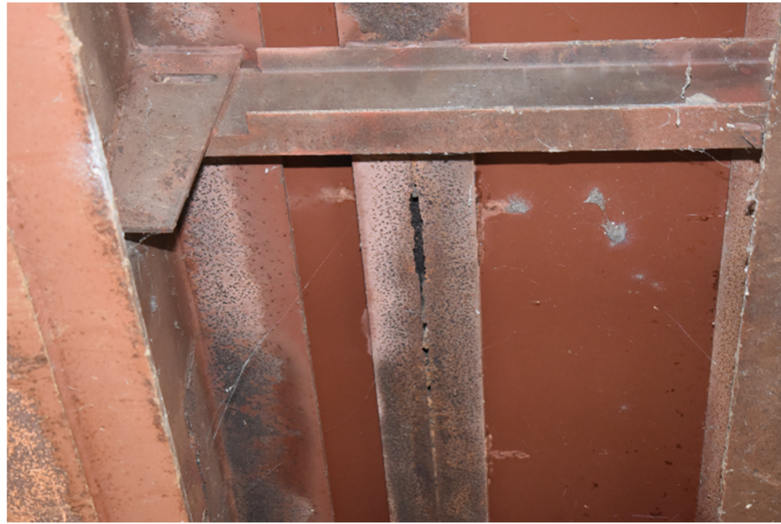
Photograph 4 – Surface corrosion of secondary stringers
