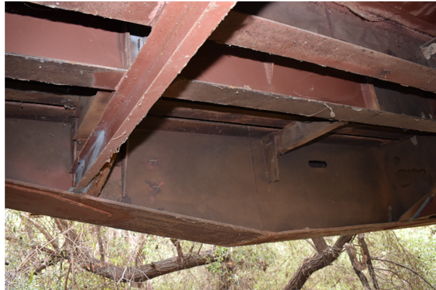
Photograph 5 – Structural members intact and undeflected
