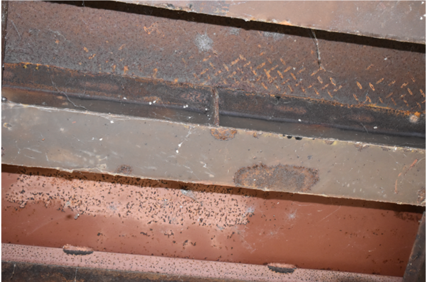
Photograph 3 – Minor stains and discoloration
